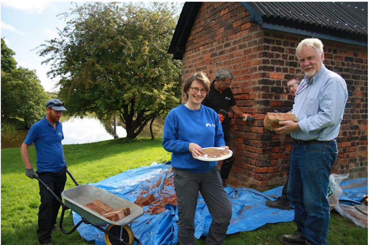
Canal & River Trust staff and volunteers renovate a historic hut on the River Weaver.
